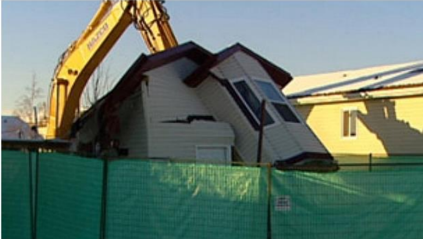
A home is demolished in Calmar, Alta. in December 2010 after a gas well was discovered leaking in the neighbourhood in 2008. (CBC)
